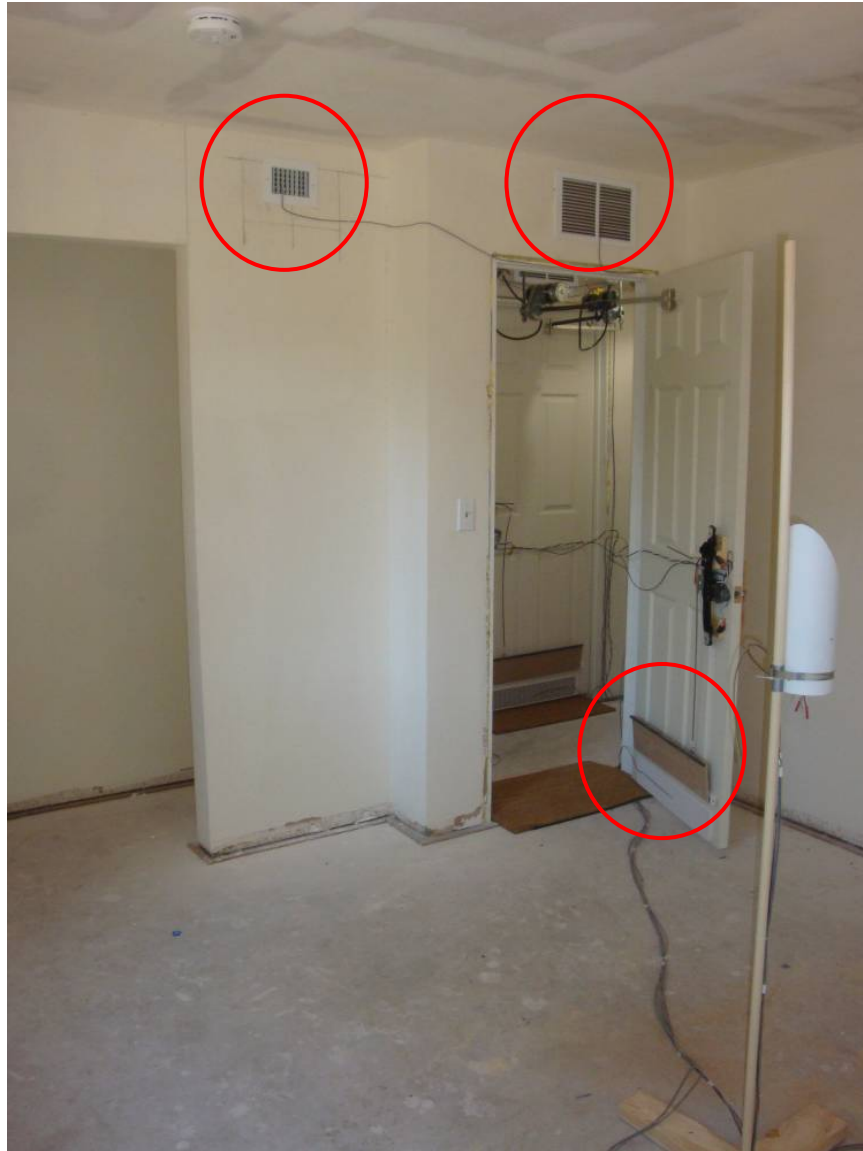
Figure 9. Typical bedroom with active forced-air register (upper left), above-door transfer grille (upper right), and bottom-of-door transfer grille (middle right)
