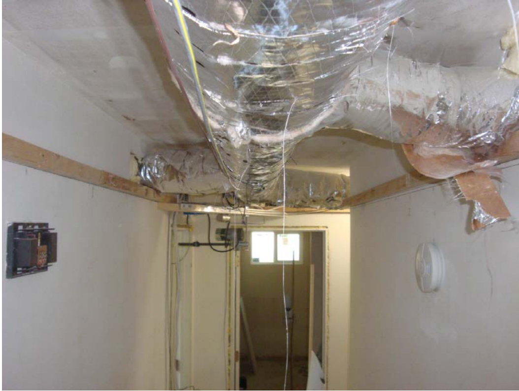
Figure 5. Test ductwork routed through the hallway and located inside conditioned space
