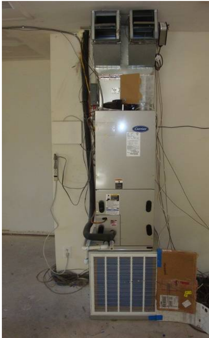
Figure 4. Test HVAC equipment installed in the living room, showing dampers to enable a single point of delivery
