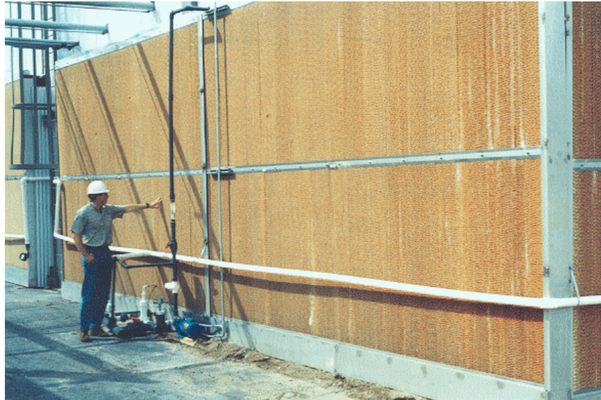
Figure 11. Setup to use packings to precool intake air at a geothermal power plant. Photo by Keith Gawlik, NREL 24495.
