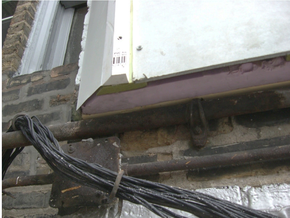
Figure 32. Base of wall with constricted access for attachment of screening (Credit: John Yi, CEDA)
