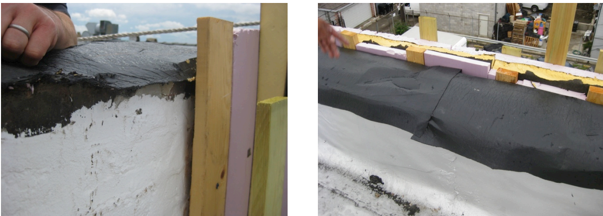
Figure 30. (L) Transition membrane not connected to elastomeric coating at face of wall; (R) transition membrane not adhered to roof membrane at inside face of parapet
