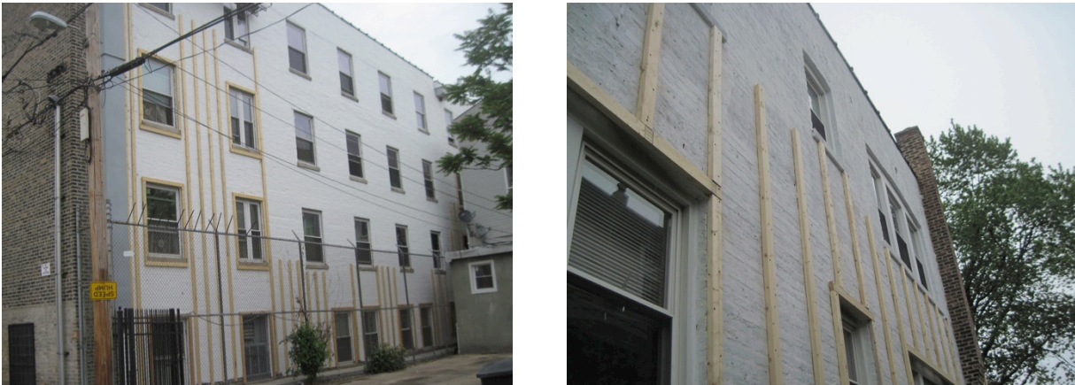
Figure 19. (L) Framing installed at in a vertical orientation only in the field of the wall. Each window opening is picture framed with the framing material. (R) Framing installed against masonry at two-family building with horizontal framing at top of window openings but in a vertical orientation elsewhere. (Credit: Scott Sanders, CEDA)
