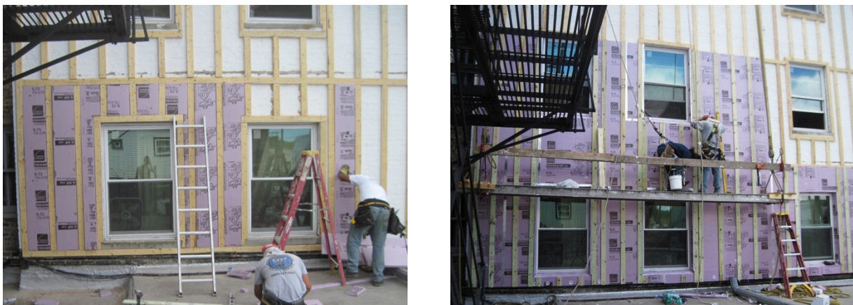
Figure 21. (L) Crews installing rigid insulation between furring; (R) second layer of rigid insulation installed over same section of wall as shown at left. Photo taken 1½ hours after photo at left. Finished first floor insulation extends another three window bays to the right of the image. (Credit: Scott Sanders, CEDA)
