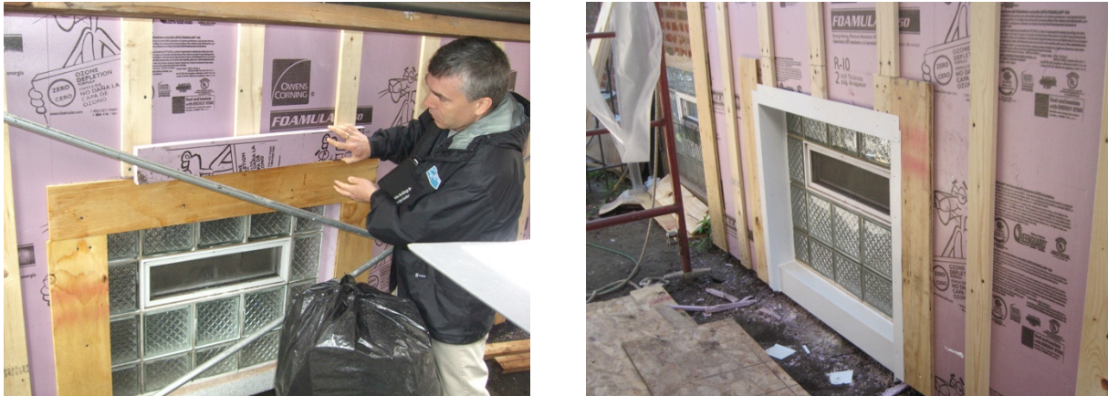
Figure 25. (L) BSC personnel explaining the attachment of trim to vertically oriented strapping; (R) the same window after the contractor reconfigured the strapping (Credit: John Yi, CEDA [L] and Scott Sanders [R], CEDA).
