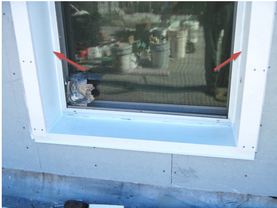
Figure 37. Return trim at the larger building butting into the vinyl window frame
