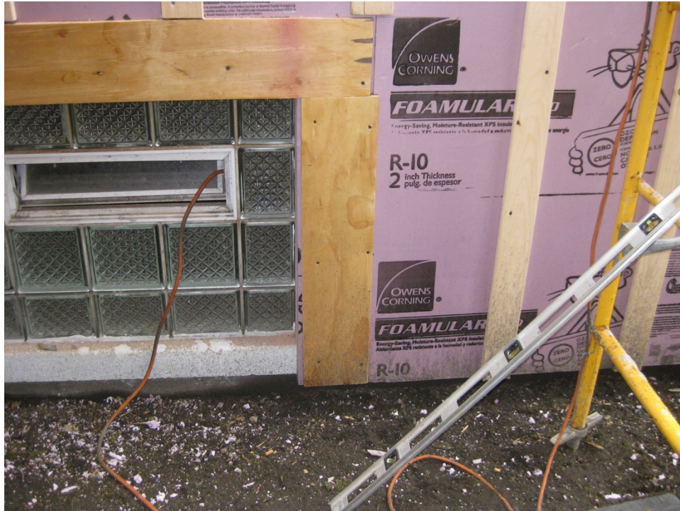
Figure 33. Base of wall insulation and over-clad assembly very close to grade at the two-family building
