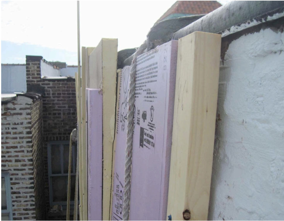
Figure 26. Beveled roof insulation used to true new cladding attachment at top of wall. Note that fasteners are left loose at the time of this photo. (Credit: Scott Sanders, CEDA)
