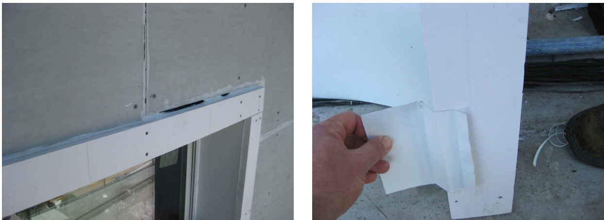
Figure 46. (L) Window head casing with no drip cap and sealant gaps; (R) Contractor project manager reviewing the drip cap flashing with the crew
