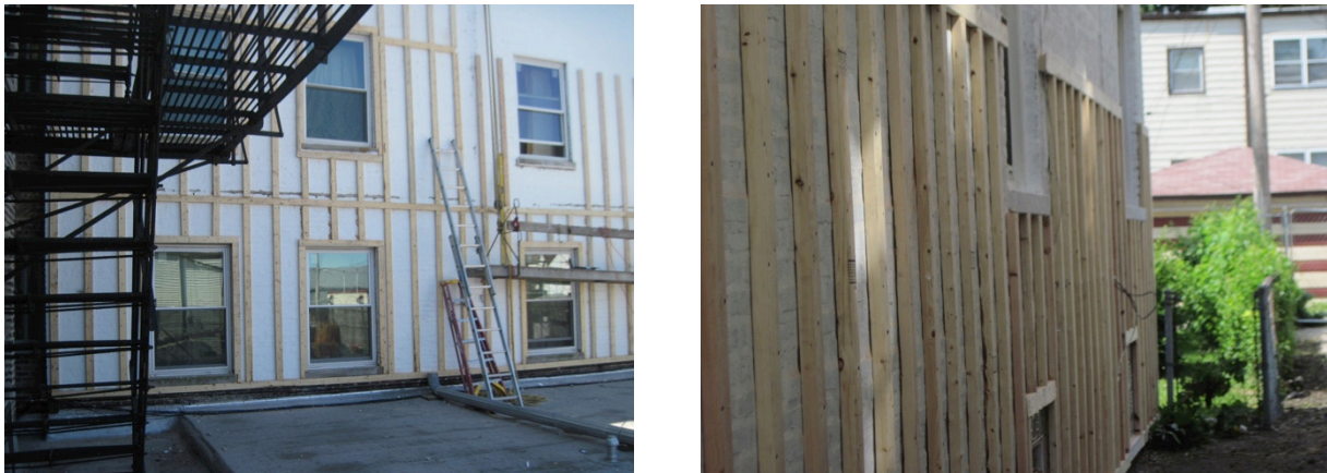
Figure 18. (L) Framing installed in a vertical orientation at 16 in. o.c. as well as horizontally at 8-ft increments in the field of the wall. Each window opening is also picture framed with the framing material; (R) Framing installed against masonry at two-family building with horizontal framing at top of window openings and at 8-ft vertical increments. (Credit: Scott Sanders, CEDA)
