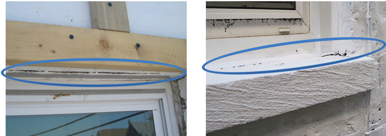
Figure 17. (L) Gap between masonry and lintel; (R) gaps at joints where sealant had not been applied as a substrate for the elastomeric paint (Credit: Scott Sanders, CEDA)
