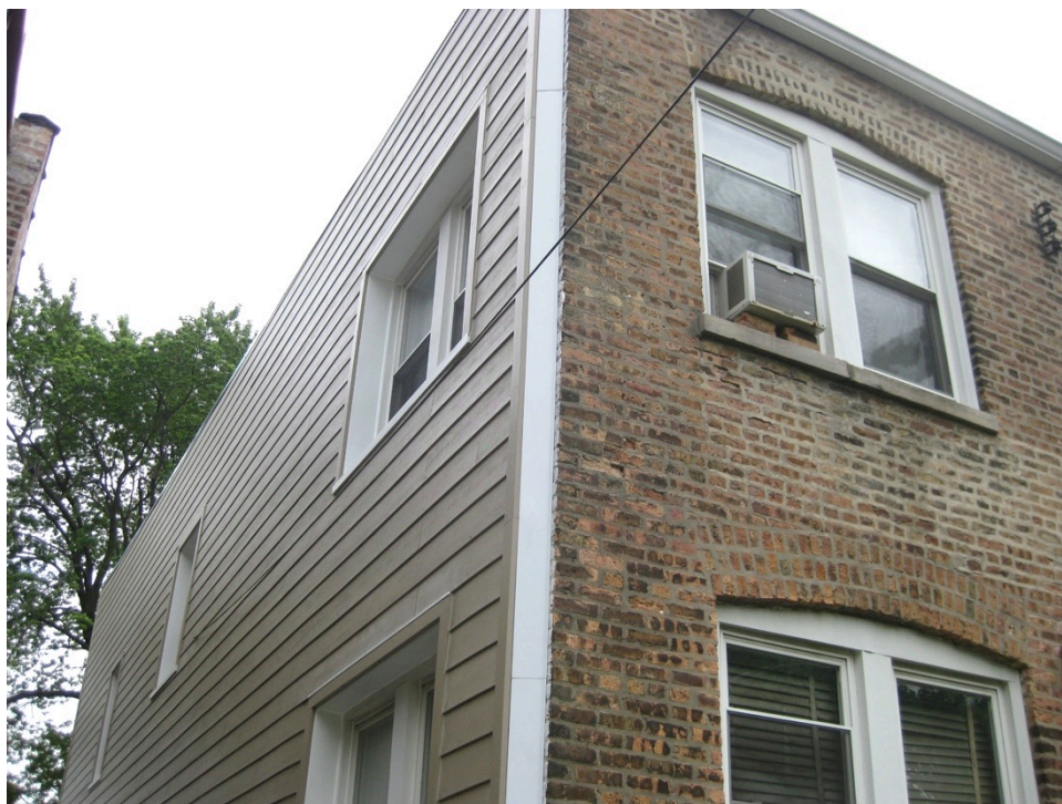
Figure 49. Treated wall at the smaller building striking a contrast with the untreated wall at the rear of the building
