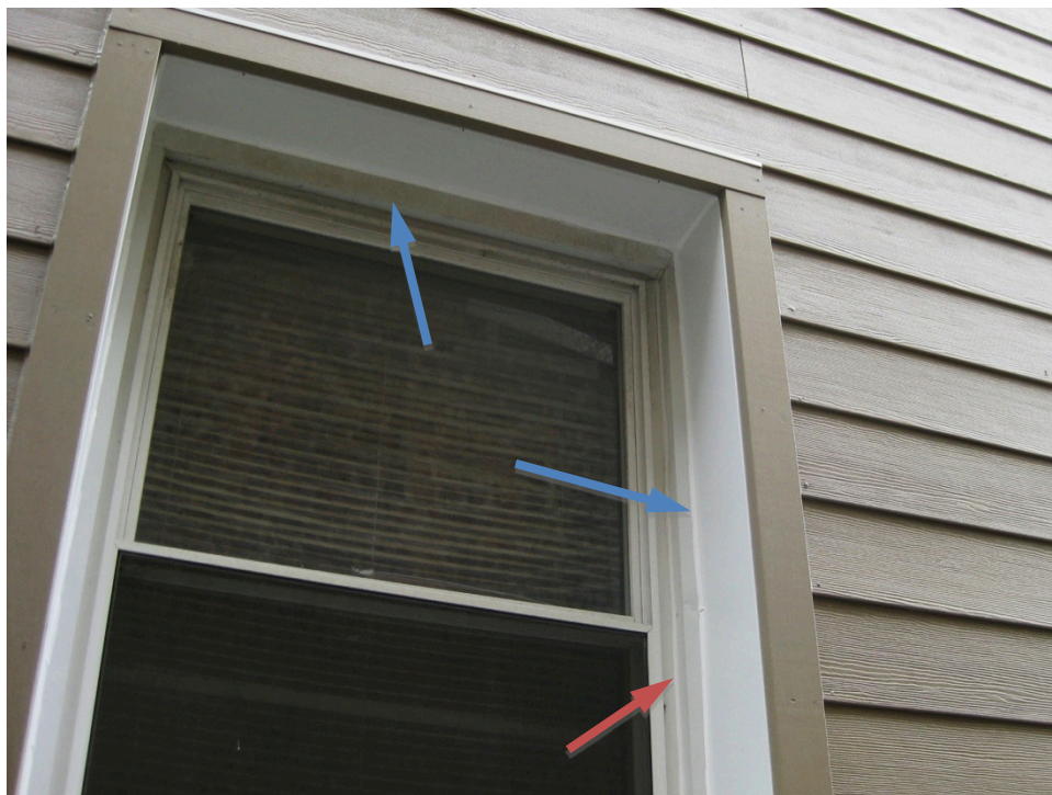
Figure 38. Return trim at the smaller building butting into the metal-clad trim surround (blue arrows) leaving the joint around the vinyl window frame exposed (red arrow)
