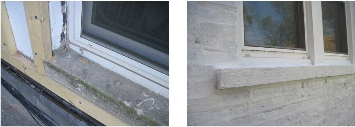
Figure 14. (L) Elastomeric paint application not complete around windows and portions of masonry surface obscured by wood framing; (R) elastomeric paint application at the two-family building covering the window sill and lapping onto the window frame (Credit: Scott Sanders, CEDA)
