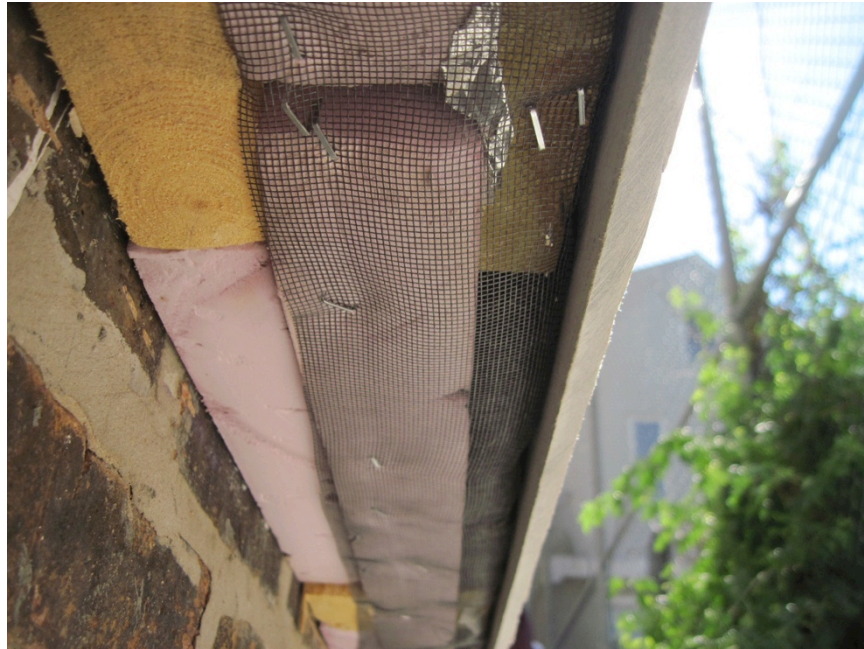
Figure 62. Screening at the base of the wall that fails to protect the exposed edge of the insulating sheathing near grade (Credit: Scott Sanders, CEDA)
