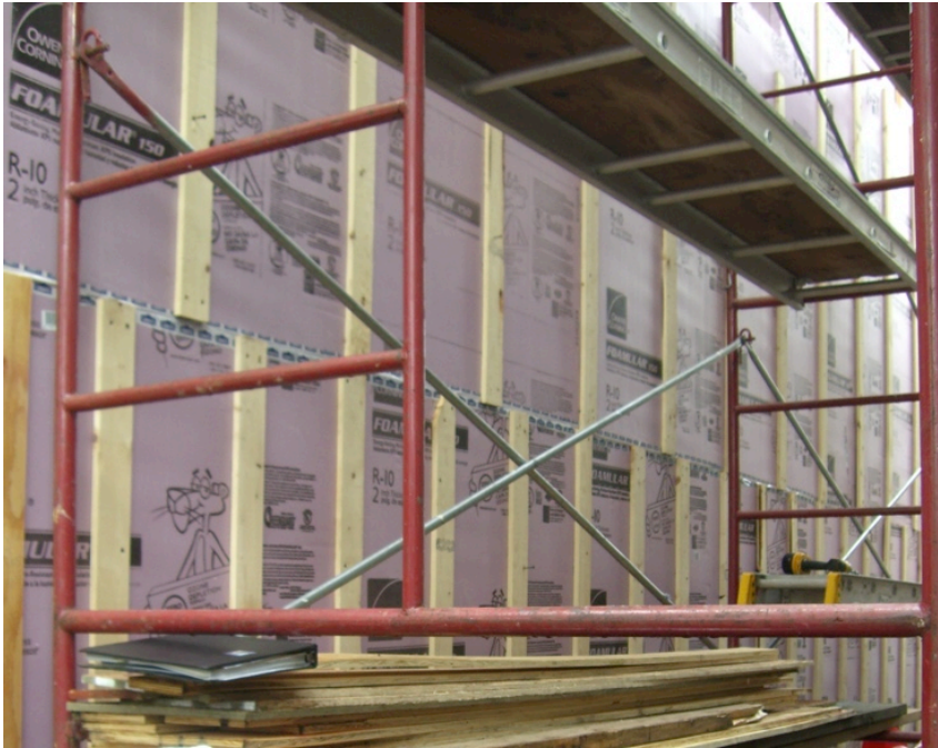
Figure 20. Strapping over insulating sheathing showing switch from 16 in. o.c. to 24 in. o.c. at the two-family building (Credit: John Yi, CEDA)
