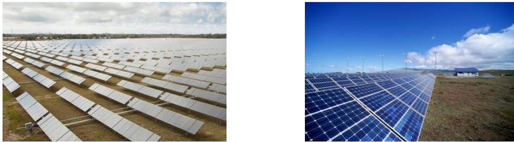
Figure 3. Mono- and poly-crystalline solar panels. Photos by (left) SunPower Corporation, NREL 23816 and (right) SunPower, NREL 13823
