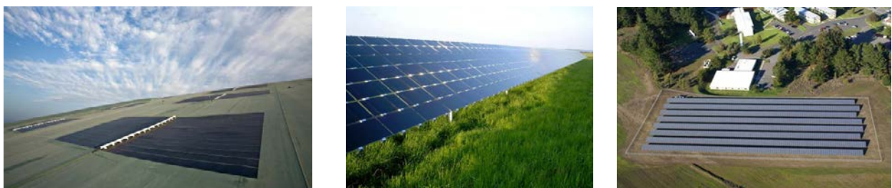
Figure 4. Thin-film solar panels installed on (left) solar energy cover and (middle/right) fixed-tilt mounting system. Photos by Republic Services, Inc., NREL 23817, (middle) Beck Energy, NREL 14726, and (right) U.S. Coast Guard Petaluma Site, NREL 17395
