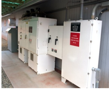
Figure 5. String inverter. Photo by Warren Gretz, NREL 07985
