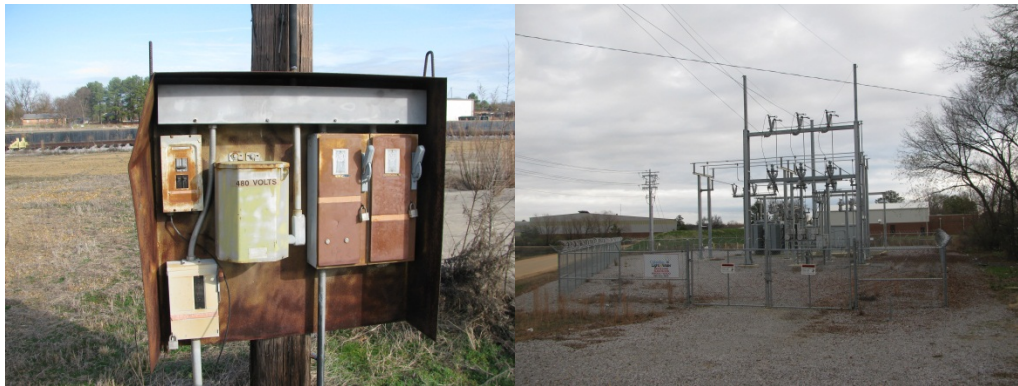
Figure 8. Electrical tie-in point for the PV system at the Kerr McGee site
