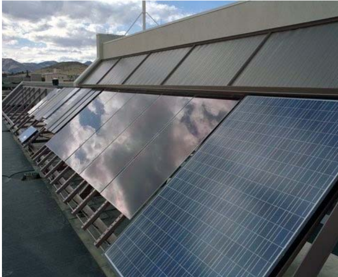
Photo by Warren Gretz, NREL/PIX 03877
