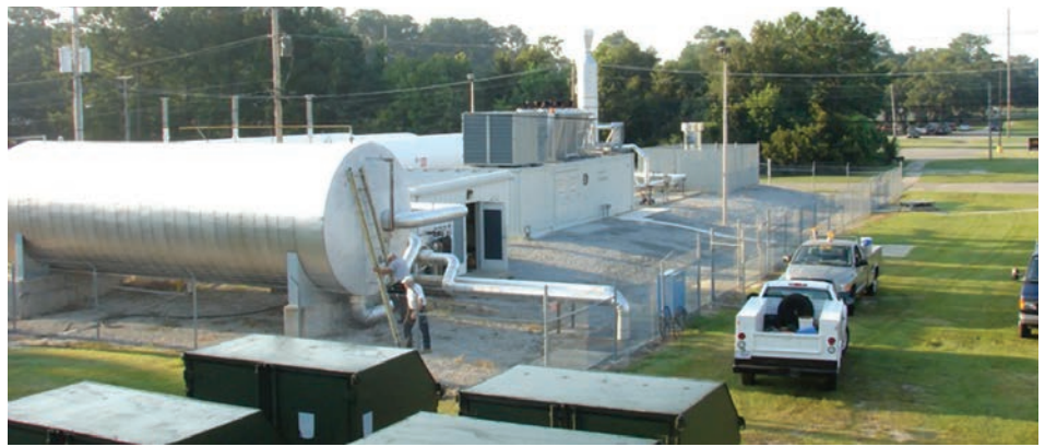
An ESPC was used to install a 1 MW cogeneration plant that supplies heat to the barracks, mess hall, and medical facility. Photo from U.S. Marine Corps Air Station Beaufort
