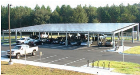
The Marine Corps’ solar roof initiative prompted the addition of this 65-kW solar array on a parking structure at MCAS Beaufort. Photo from U.S. Marine Corps Air Station Beaufort
