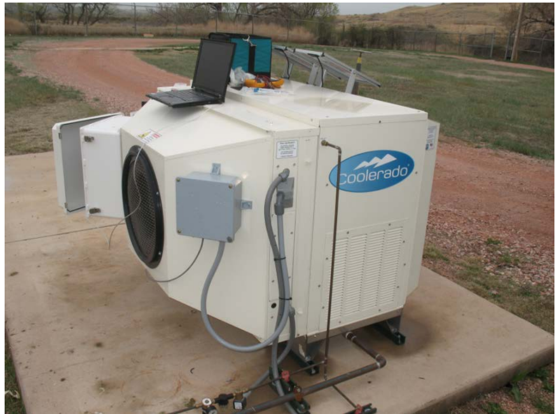
Waste Water Unit
