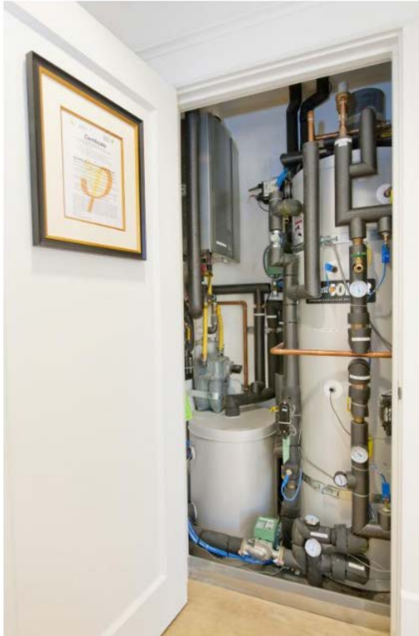
Figure 8. Mechanical closet containing solar thermal storage system and tankless water heater
