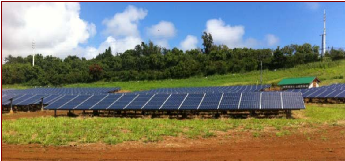
Figure 4-7: 1.2 MW DC Photovoltaic array on Kaua'i, Hawaii (Credit J. Keller, NREL)
