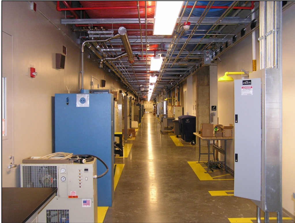
A 12 ft wide service corridor with "notches" for noise producing equipment
