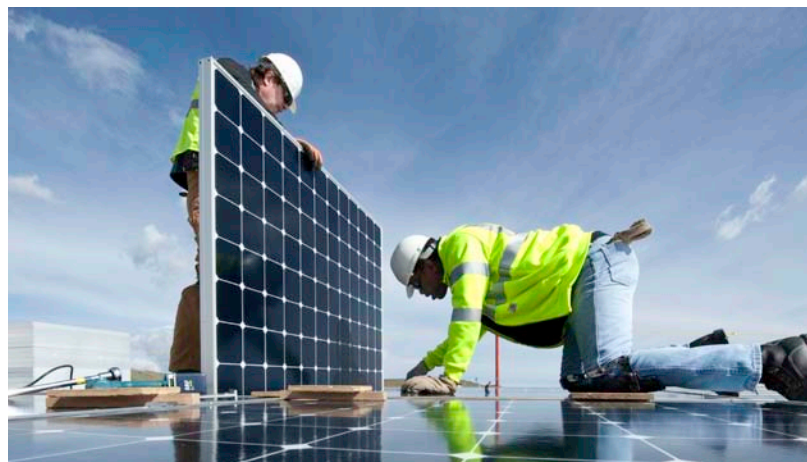
Photo by Dennis Schroeder, NREL/PIX 21499
