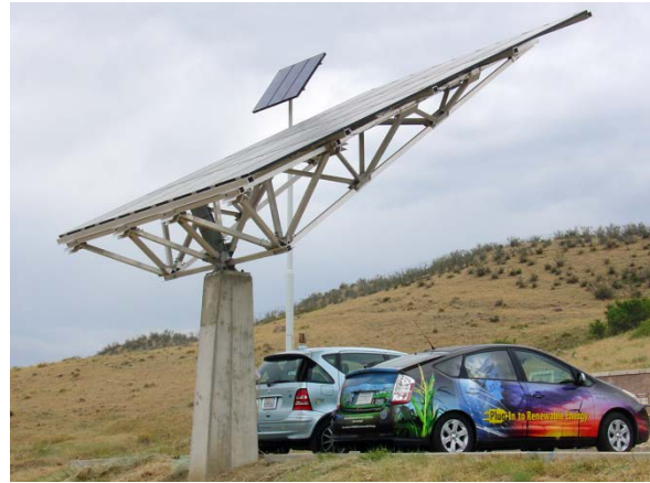
Solar Vehicle Charging Station
