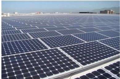
Photo from City of San Jose, NREL/PIX 19487
