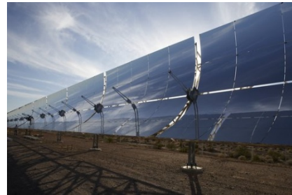
Photo by Geri Kodey NREL/PIX 14380
