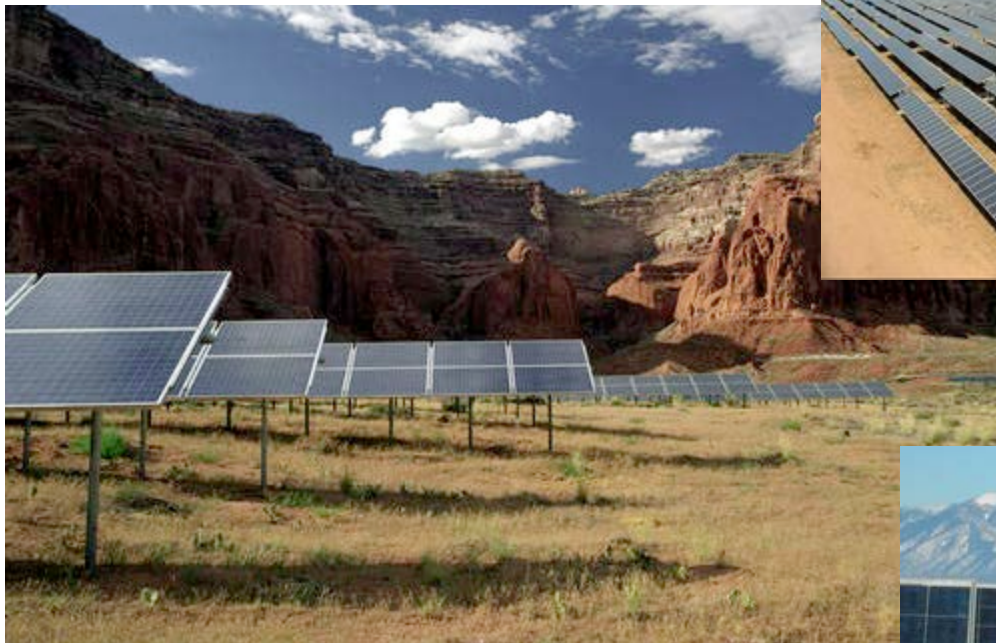
Photo by Warren Gretz, NREL/PIX 07990
