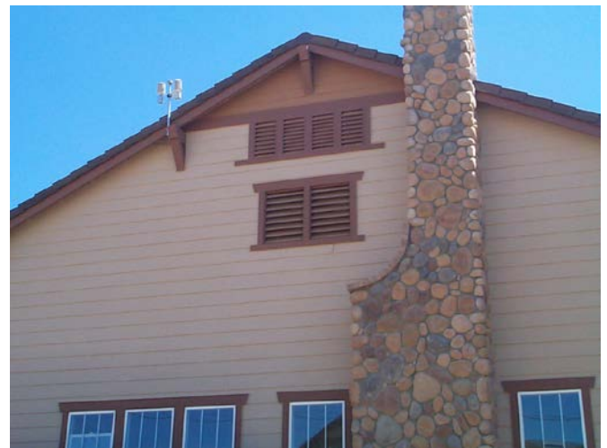
Figure 11: For this house the upper set of louvers is for the outside air intake; the lower pair is for attic ventilation.
