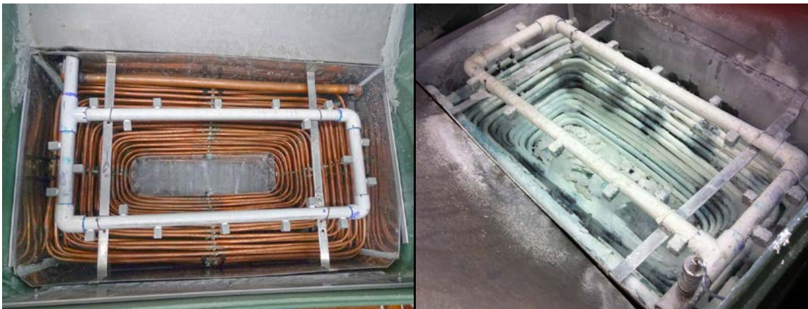
Figure 4: Condenser coil before (left) and after (right) prolonged operation without any water management strategies
