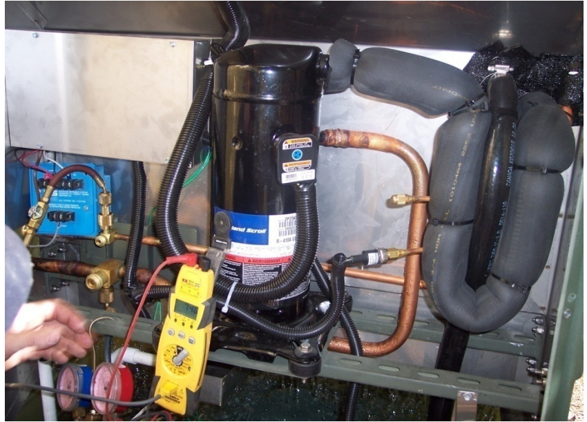
Figure 9: Gauges connected to operating evaporative condenser to verify correct charge
