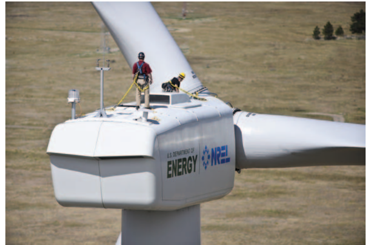
Wind technicians work on the DOE 1.5 MW turbine at the National Wind Technology Center. Photo by Dennis Schroeder, NREL/PIX 19067
