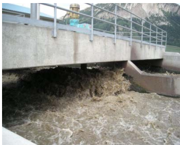
Figure 6. Mechanical aerator in oxidation ditch
