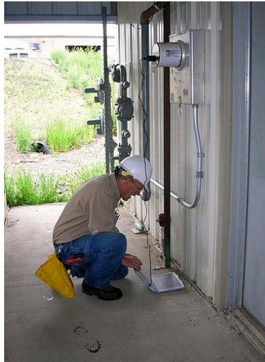
Figure 4. Collecting UV system power draw data
