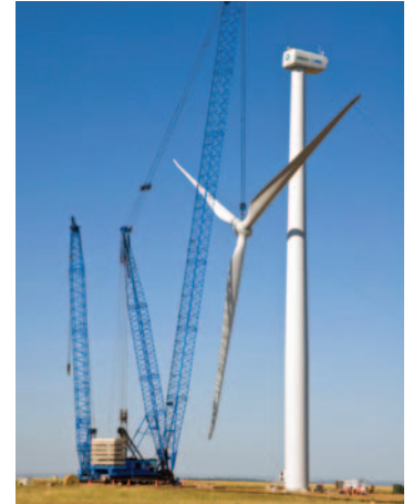
Installation of DOE's 1.5 MW GE wind turbine at the NWTC. Photo by Patrick Corkery, NREL/PIX 16569
