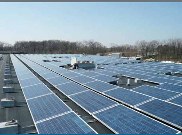
A 112-kW PV system is displayed on the rooftop of the Hankin Group in Exton, Pennsylvania. Photo from Mercury Solar Solutions, NREL/PIX18062
