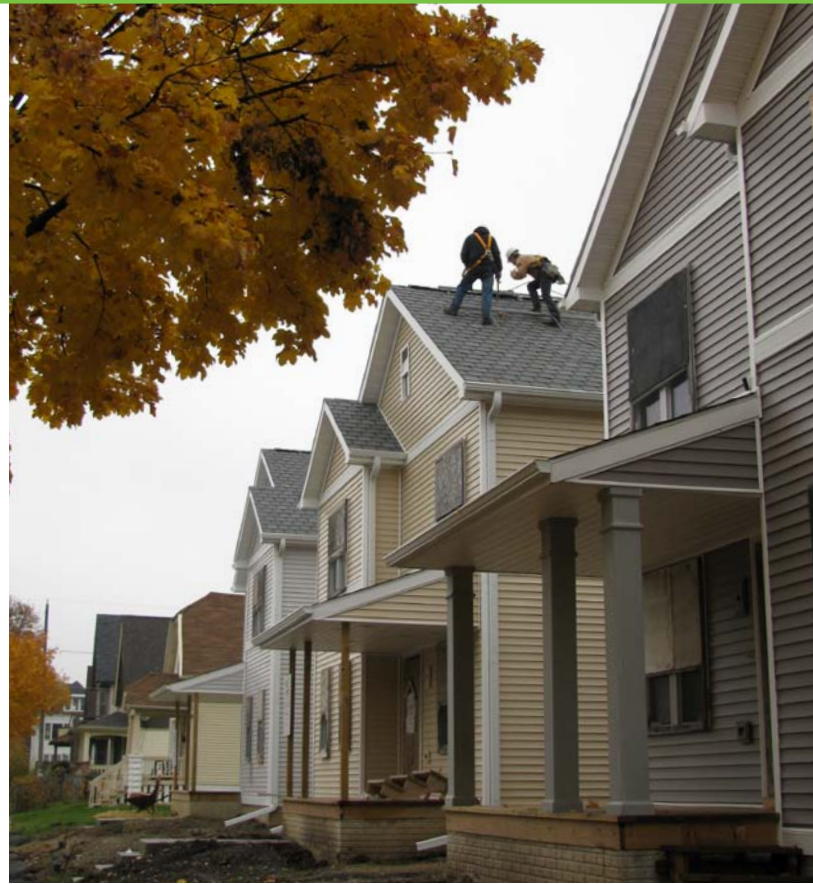
Installers get hands-on experience installing solar hot water panels on a Habitat for Humanity home. Photo from MREA, NREL/PIX 18705
