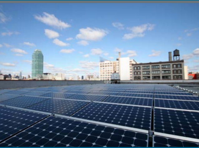
Solar Energy Systems installed this 49.1-kW solar photovoltaic system on the rooftop of the Novelty Crystal corporation in Queens, New York. Photo from Solar Energy Systems, NREL/PIX 18521
