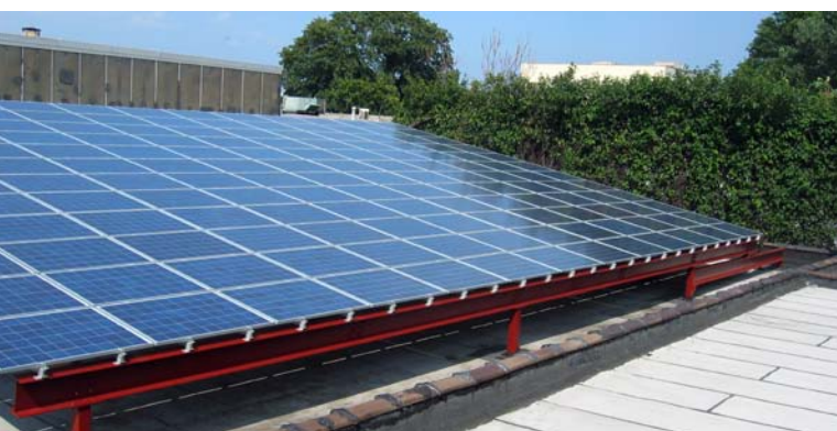
Solar Energy Systems installed this 68.4-kW solar photovoltaics system. Photo from Solar Energy Systems, NREL/PIX 18522
