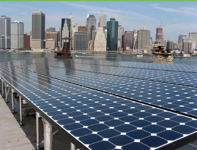
Aeon Solar installed this solar PV rooftop system in Brooklyn. Photo from Aeon Solar, NREL/PIX 18523
