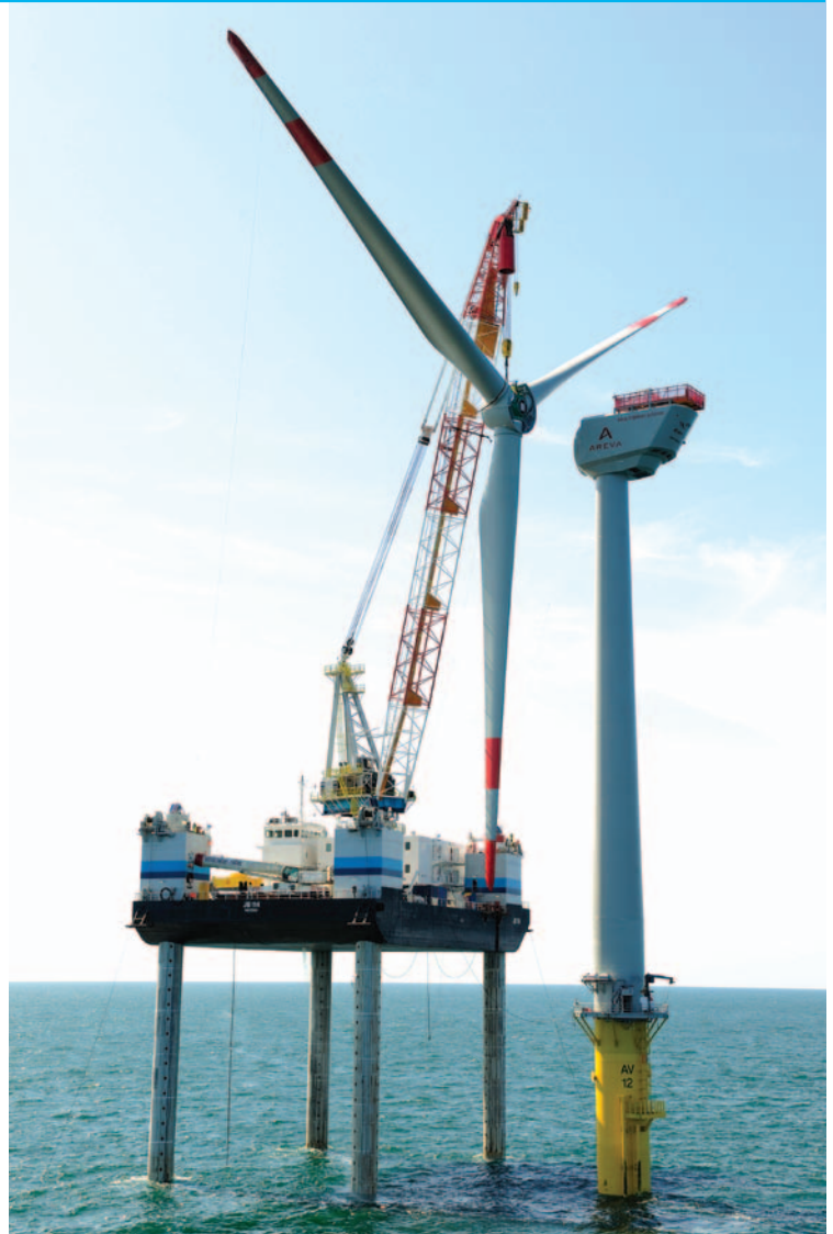
A crane mounted on a barge designed for offshore wind turbine installation lifts a rotor into place. Photo courtesy of © DOTI 2009-alpha ventus
