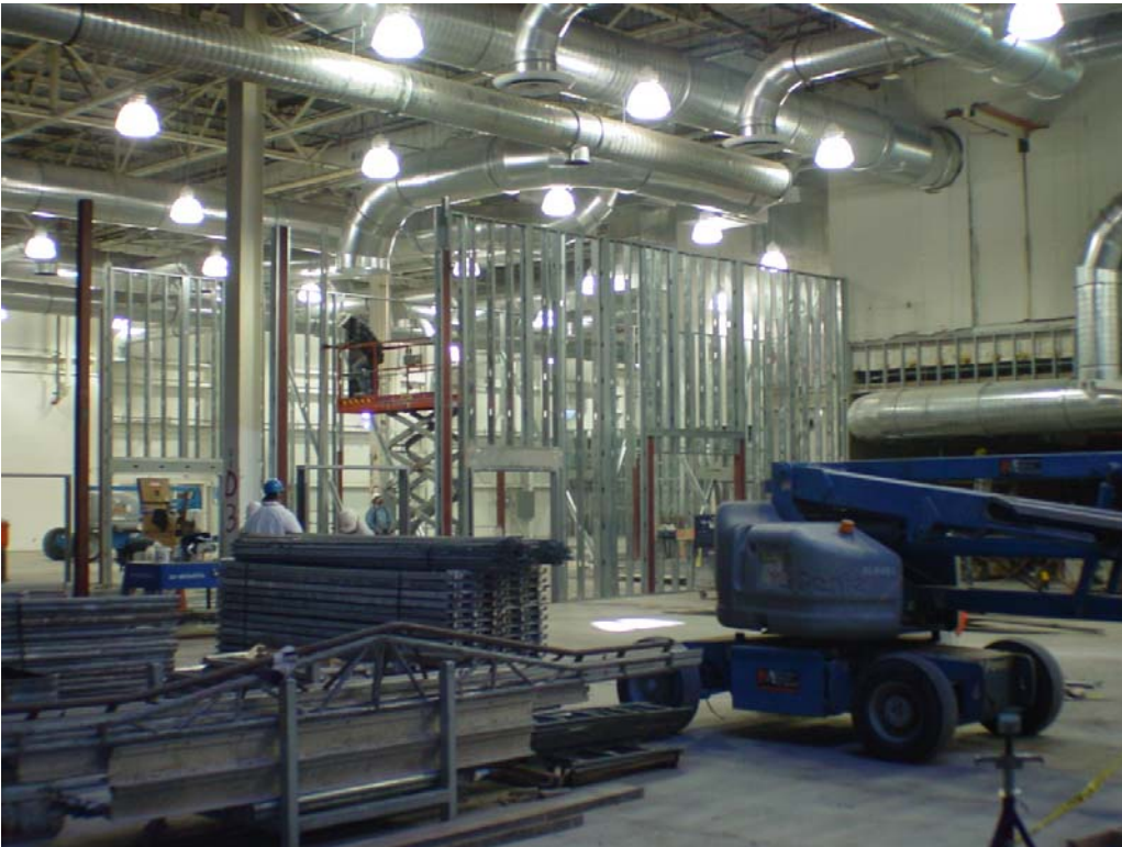
Fig. 2.5. Interior rooms, overhead lighting and HVAC under renovation in the Tucson facility. (Credit: Global Solar Energy)
