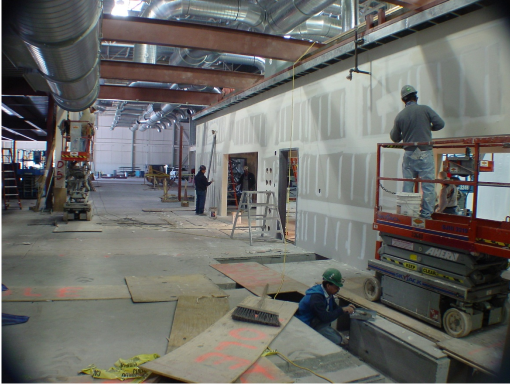
Fig. 2.4. Interior structures, equipment chases and HVAC under renovation in the Tucson facility. (Credit: Global Solar Energy)
