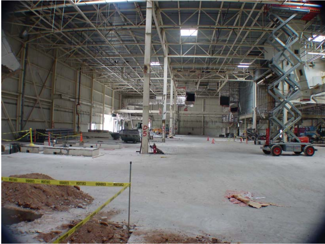
Fig. 2.2. A northeast section of the GSE Tucson building under demolition. (Credit: Global Solar Energy)
