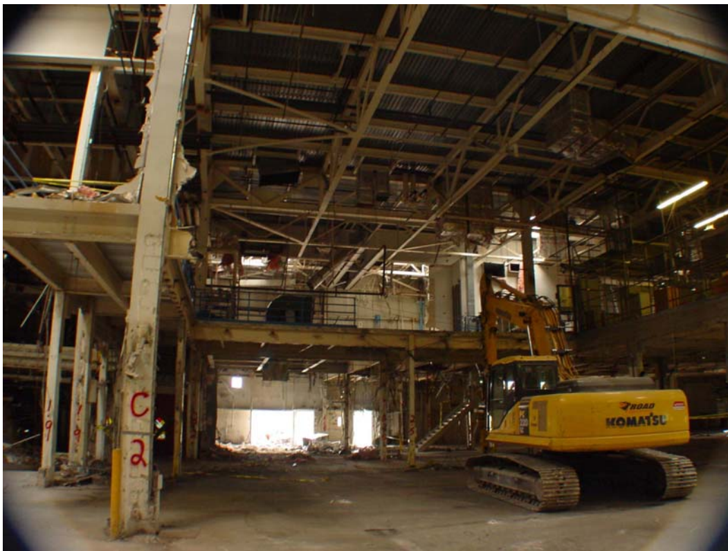
Fig. 2.1. One section of the GSE Tucson building under demolition. (Credit: Global Solar Energy)
