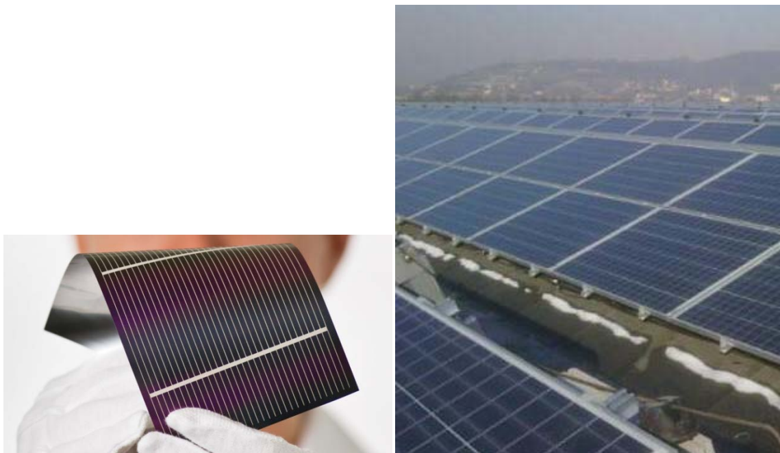
Fig. s2a,b. A “Gen2” cell at GSE (210 cm 2 ), and modules made with Gen2 cells at the largest rooftop CIGS installation in the world (820 kWp at Vincenzo, Italy). (Credit: Global Solar Energy)
