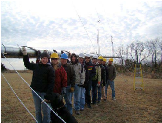
James Madison University students installing a meteorological tower in Quinby, Virginia. Photo from Jonathan J. Miles, NREL/PIX16246
