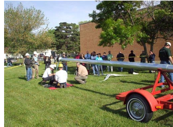
Wind turbine installed at Hope Street Academy in Topeka, Kansas. Photo from Ruth Douglas Miller, NREL/PIX17336
