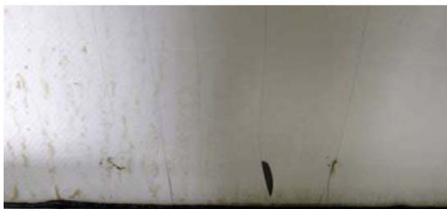
Figure 7. Hydrolytically degraded, embrittled, and cracked backsheet of model 1 after round 3 of the alternating DH+/TC sequence.
