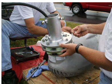
Kansas State University Wind Applications Center students learn valuable career skills by participating in project installations. PIX16024/Ruth Douglas Miller.
