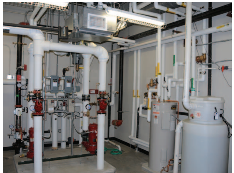
A ground source heat pump system provides heat and cooling to the 9,580-square-foot Business Incubator in Greensburg, Kansas. PIX17206
