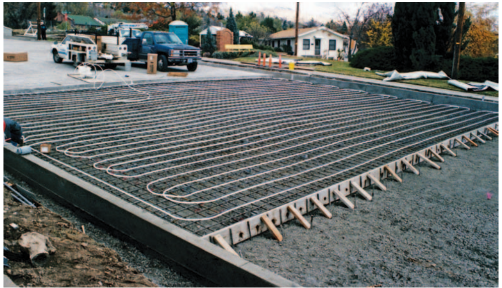
The city of Klamath Falls, Oregon, uses low-temperature geothermal resources for district heating applications such as this snowmelt tubing installed in slurry backfill under sidewalks. The City uses the system to melt snow on more than 50,000 of its sidewalks and crosswalks. PIX08831
