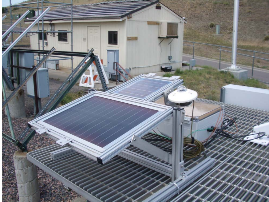
Figure 3-2. BP Solar model SX5M (top) and UNI-SOLAR model US-11 (bottom) PV modules with plane-of-array pyranometer at NREL for June 7-9, 2008. PV modules are south-facing and tilted 12^\circ from the horizontal. The enclosure behind the PV modules contains the data logger.
