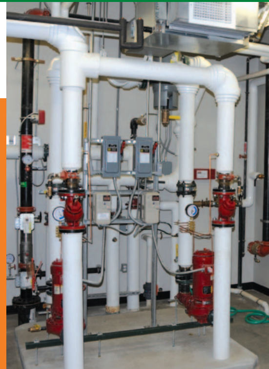
The geothermal heat pump system provides heating and cooling to the building.
