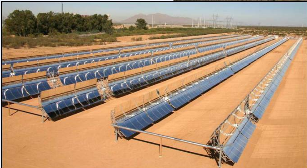
1-MW Arizona Trough Plant – near Tucson, AZ - 2006
