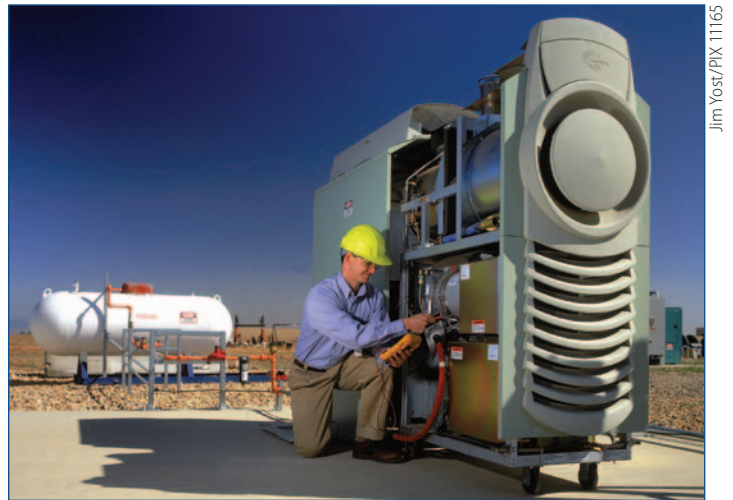
30-kW micro-turbine powered by propane at the DER Test Facility.
