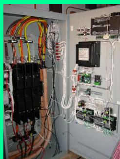
Switchgear, Relays, & Controls
