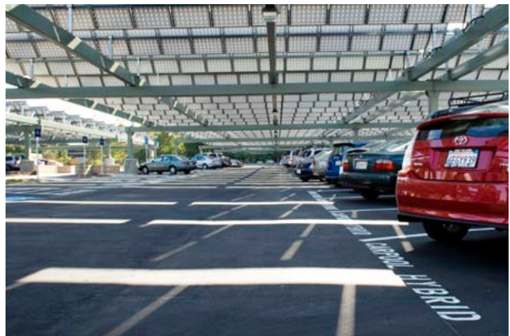
The parking lot solar plant provides shade for employee vehicles while generating substantial power.
