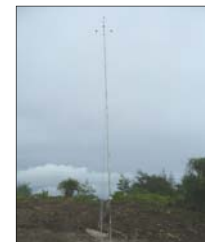
60-m Met tower installation at Naval Magazine on ridgeline in western Guam. Installation by DNV-GEC.
