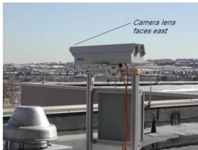
Fig. 3: CC640 digital camera from Campbell Scientific, Inc., located on building roof.
