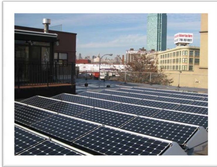
Figure 11. View of the Rooftop PV System (Black Bear Co.)
