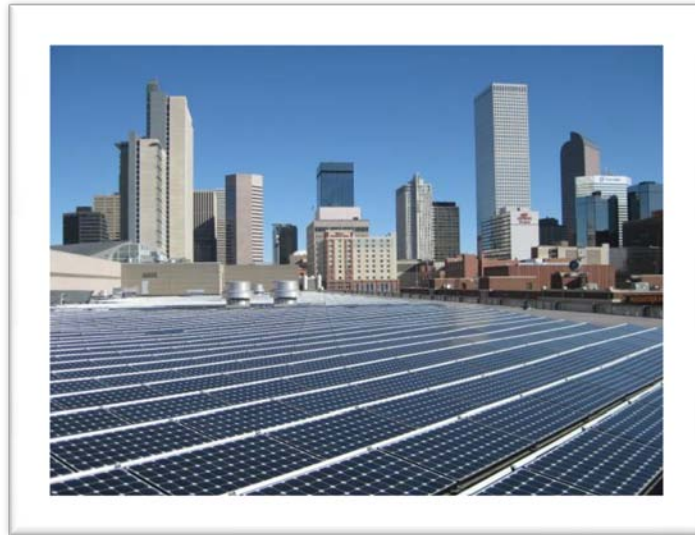
Figure 15. Colorado Convention Center PV System
