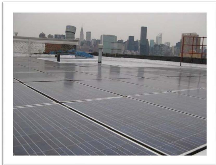
Figure 13. Rooftop PV Systems at GMDC
