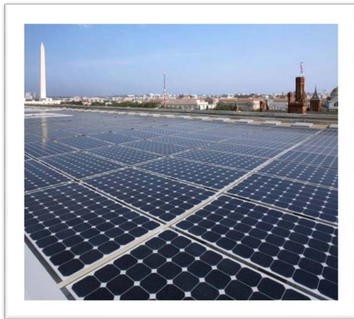
Figure 6. PV Array on Forrestal Building
