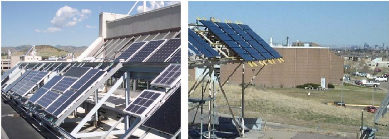
Figure 1. Digital images of the PERT modules at left, looking west; and HVST2 modules at right, viewed east, at the OTF.
