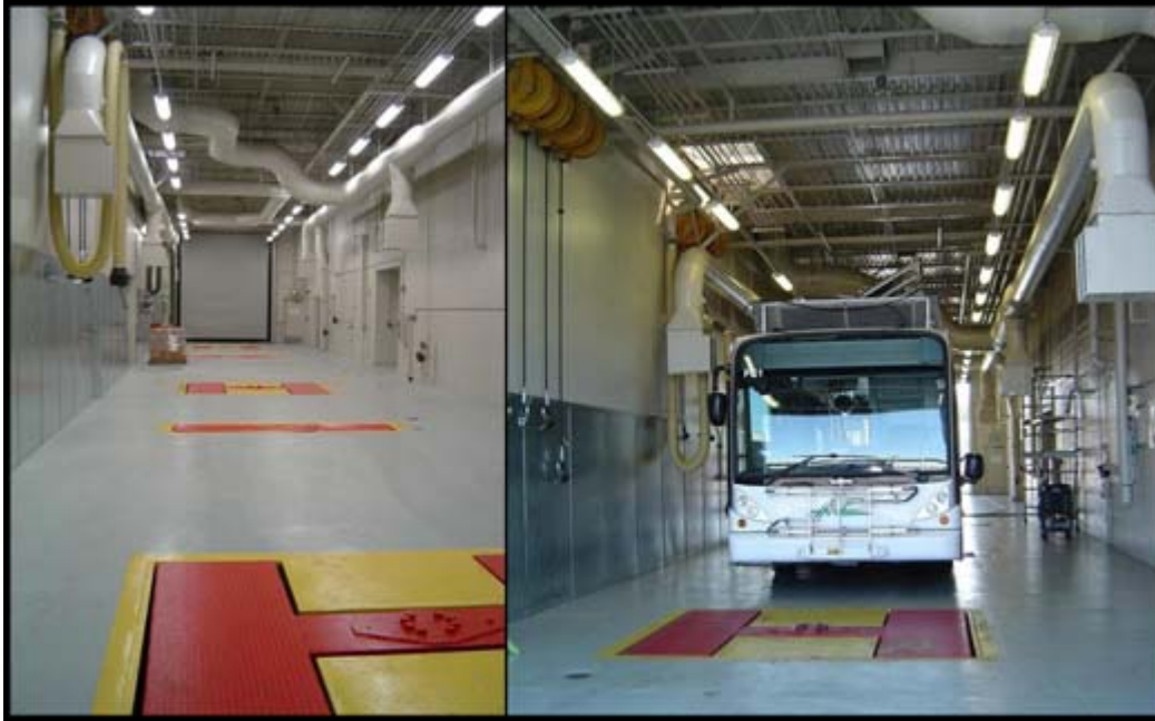
Figure C-6. Modified maintenance bay at AC Transit East Oakland Division
