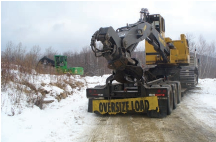
Road construction begins on the Lempster Wind Project. (Photo credit: Iberdrola Renewable Energies USA/PIX15574)
