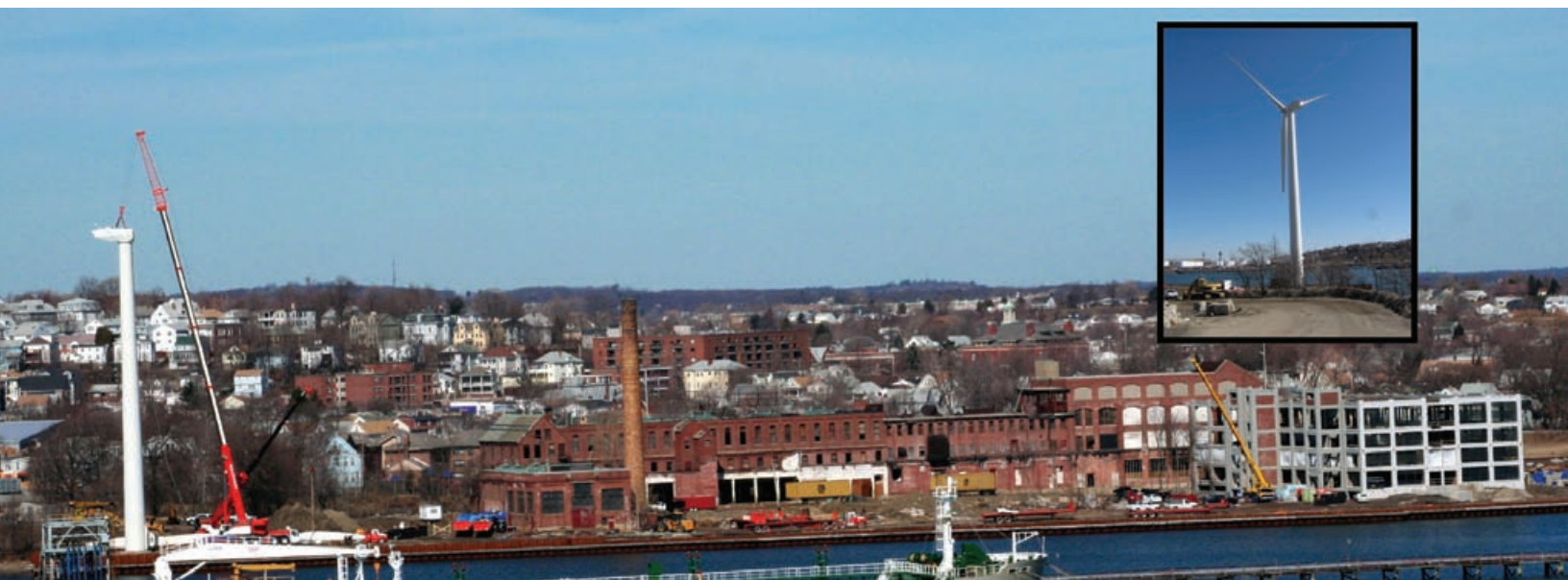
A panoramic view of the nacelle for a 600-kW wind turbine being lifted atop the tower at Forbes Park in Chelsea, Massachusetts. Inset: The installation is complete! (Photo credit: Boreal Renewable Energy Development/PIX15573)
