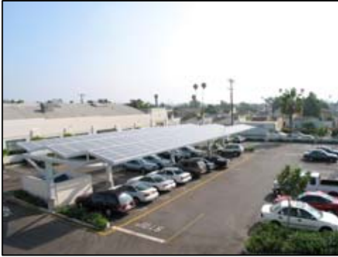
Solar car park. Courtesy of Solar Electric Vehicles
