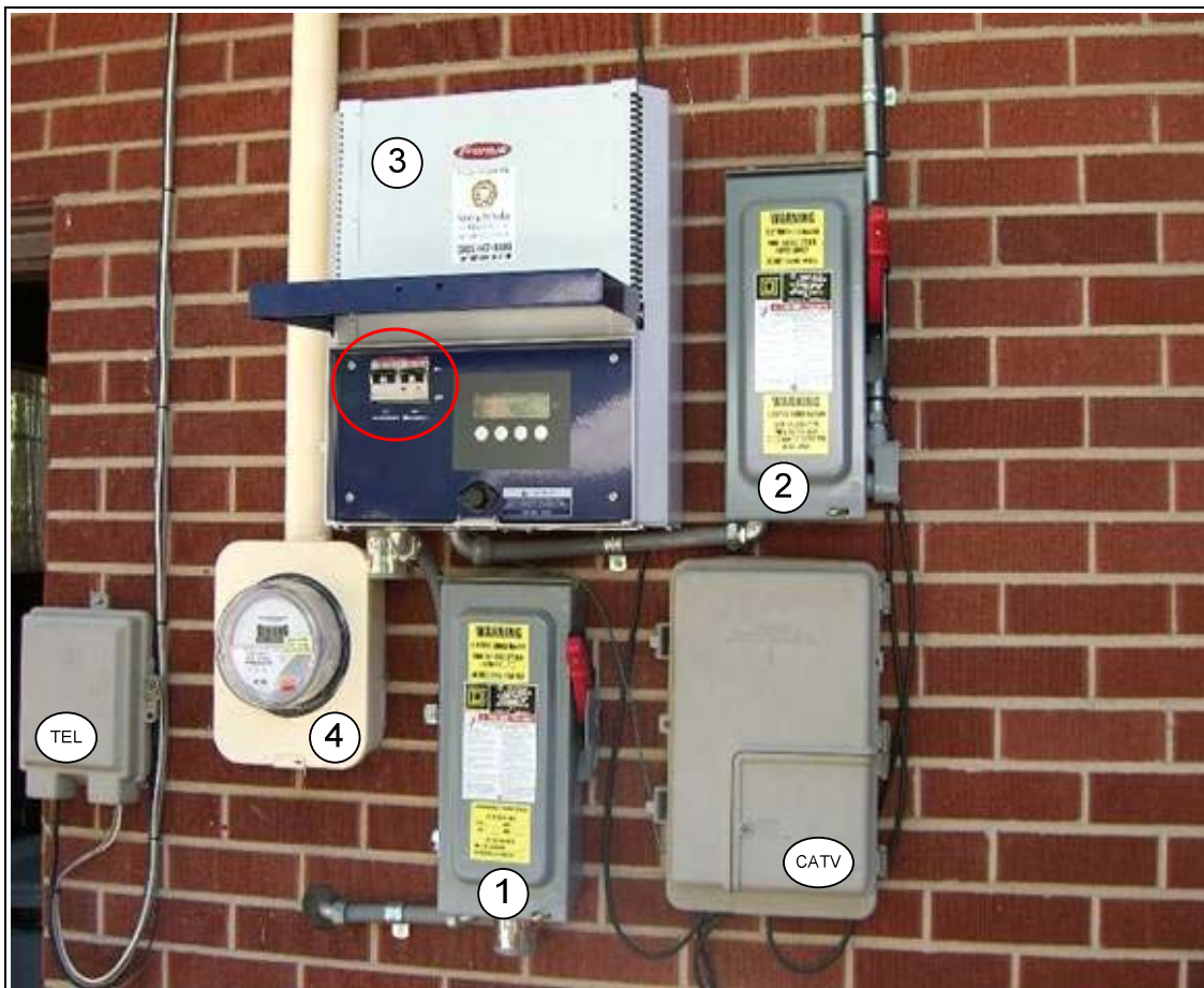
Figure 2. A typical residential PV installation includes (1) an EDS, (2) a DC disconnect, (3) an Inverter (with AC and DC breakers shown in the red circle), and (4) a revenue meter
