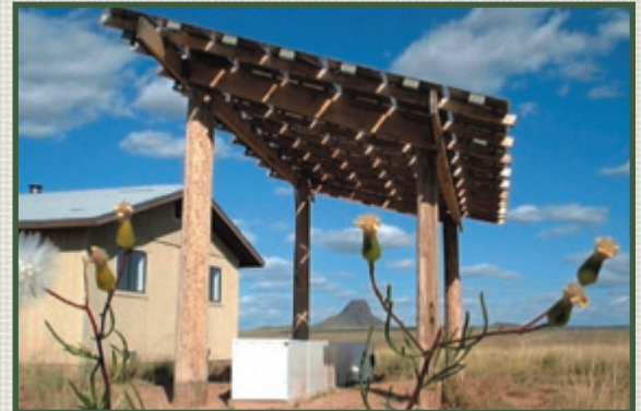
Solar electric array on Navajo home
