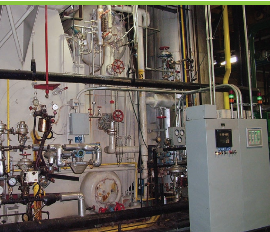
The steam system at Goodyear's Union City plant is served by four dual fueled (natural gas and No. 6 fuel oil) boilers, such as the 60,000 lbs/hr boiler pictured above.
