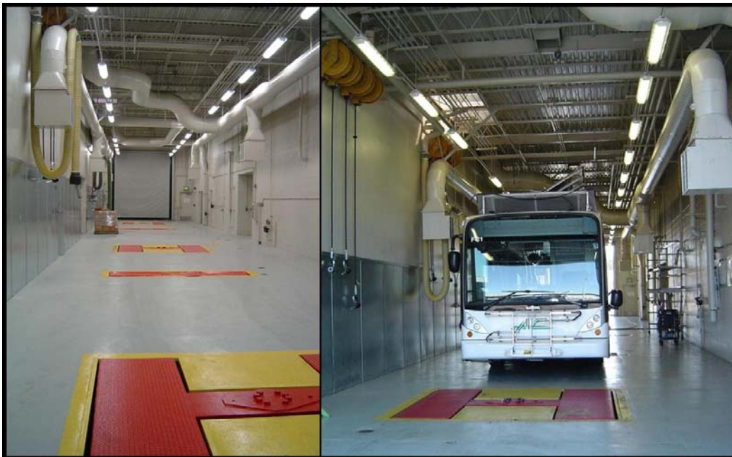
Figure 5. Modified maintenance bay at AC Transit East Oakland Division
