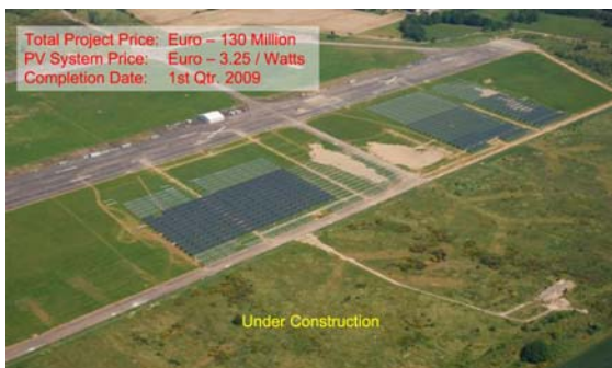
Figure 4: A 40-MW thin-film CdTe solar field being built in Saxony, Germany to be completed in early CY 2009
