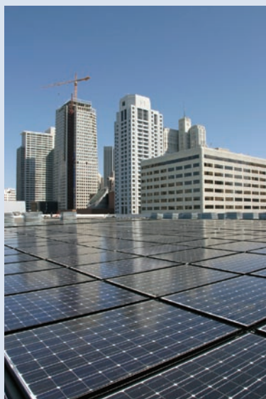
This 675-kW photovoltaic array on the Moscone Center in San Francisco, CA, converts sunlight directly into electricity. Credit: PowerLight Corporation.
