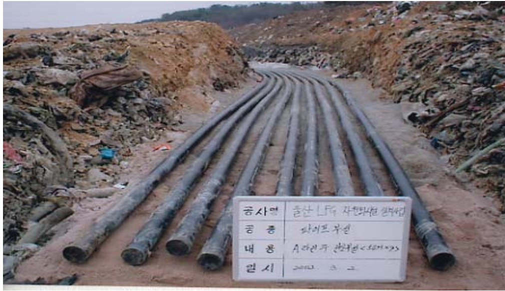
Figure 3: Pipelines for transporting captured LFG from landfill to adjoining LFG treatment facility
