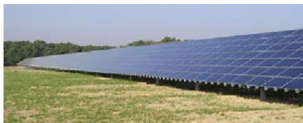
Fig. 1. First Solar's 1400-kW thin-film CdTe solar field deployed in Germany.
