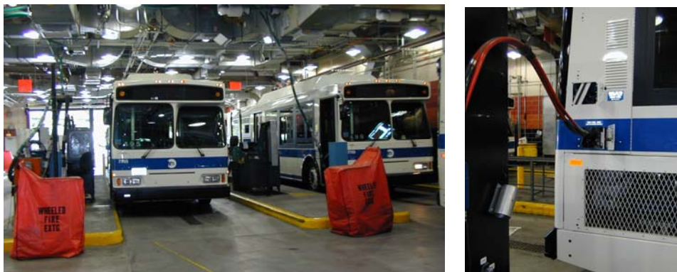
Figure 3. CNG Fuel Lanes at West Farms Depot
